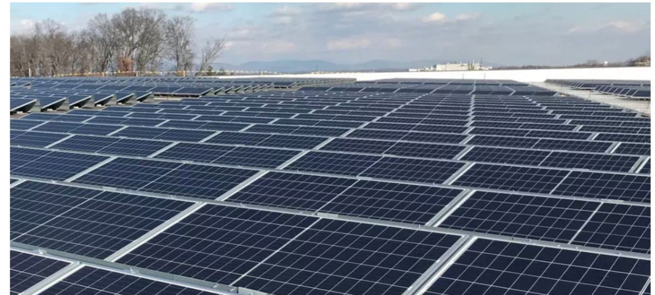
Roof mounted PVs
