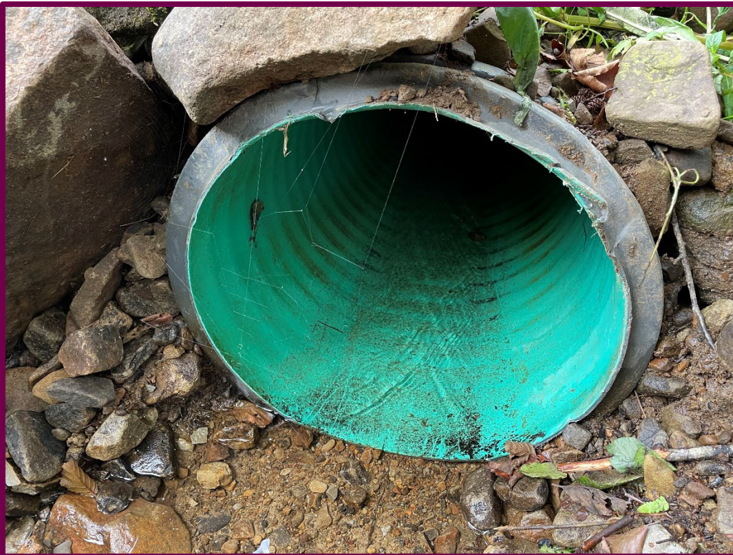
Figure 16: Watercourse piped under track located to the east of the proposed site
